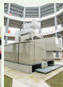
In-house power generation facilities
