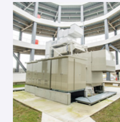
In-house power generation facilities
