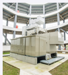
In-house power generation facilities
